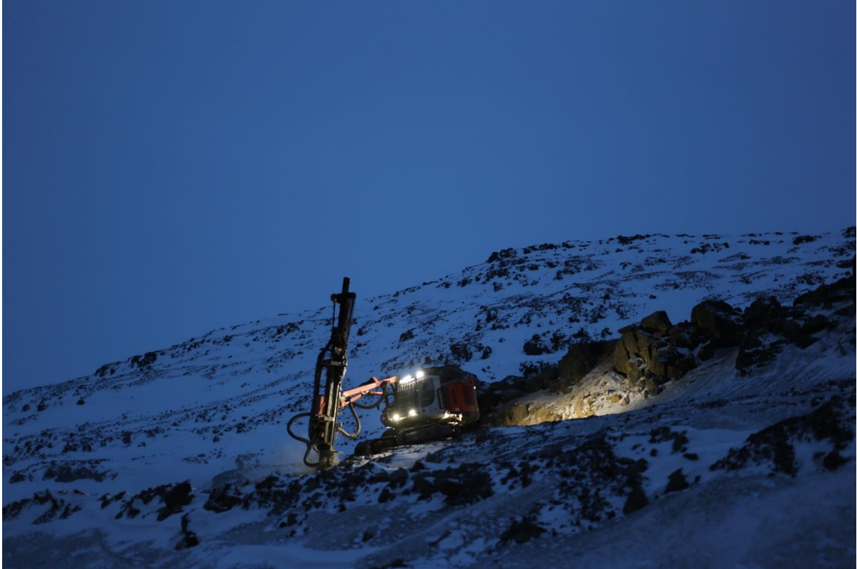
Figure 2.7: Photograph of the road to Patreksfjörður under repair during winter. The mountain roads are key to connectivity in the southern Westfjords (Photograph by author).
