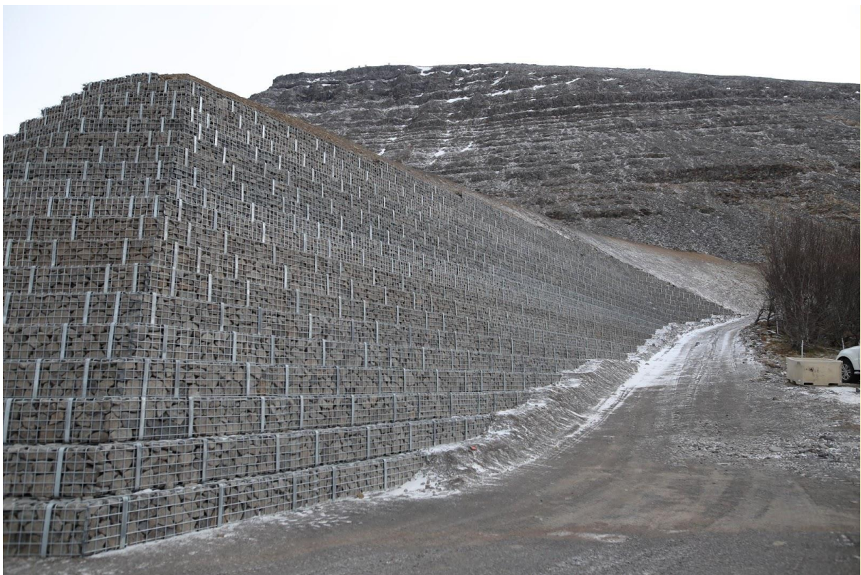
Figure 2.12: The avalanche barrier at Urðargata. Photograph of one of the avalanche barriers under construction in Patreksfjörður, with the mountainside behind it (photograph by author)
